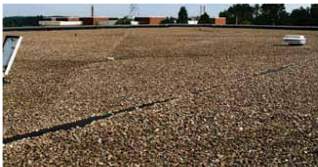
The 29-year-old EPDM roof protecting the Jamerich Building at Northern Michigan University in Marquette, Mich., is still performing well.
